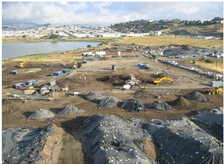
Overview photo IR-02 (foreground) and adjacent PCB Hot Spot. Photo shows excavations, radiological screening conveyor systems and stockpiles. The Hunters Point 'landfill' is in the upper right corner and the San Francisco Bay is to the left.
